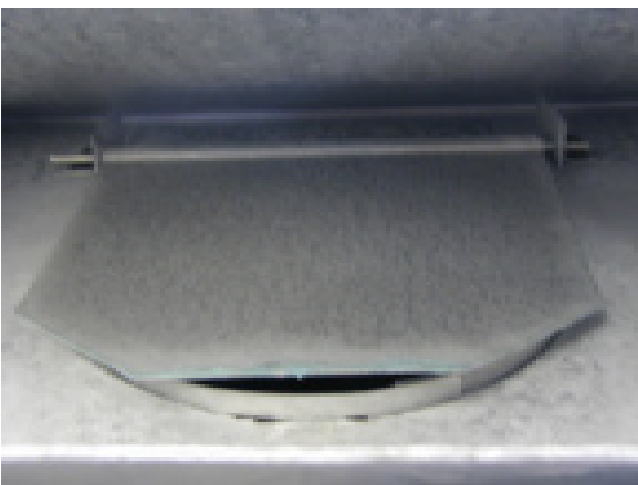
Fig. 11B Improperly closed backdraft flapper
